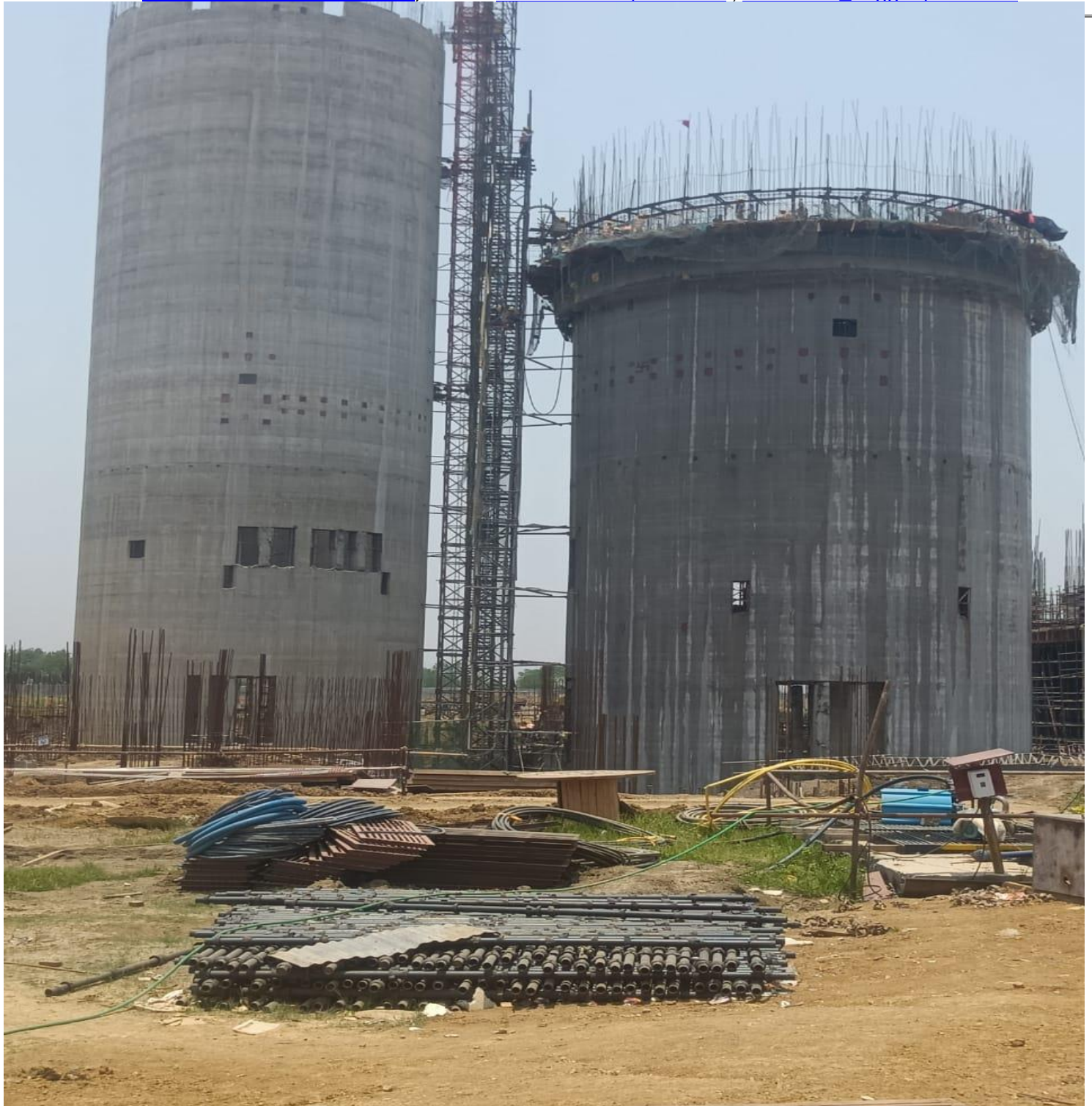
18.8 Mtr Dia, 52 Mtr Ht. 1 No of Cement silo At. Baloda Bazar, Chattisgarh. Client: - Ultra Tech Cement
